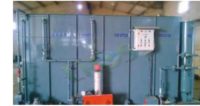
Sewage Treatment Plant (STP)
